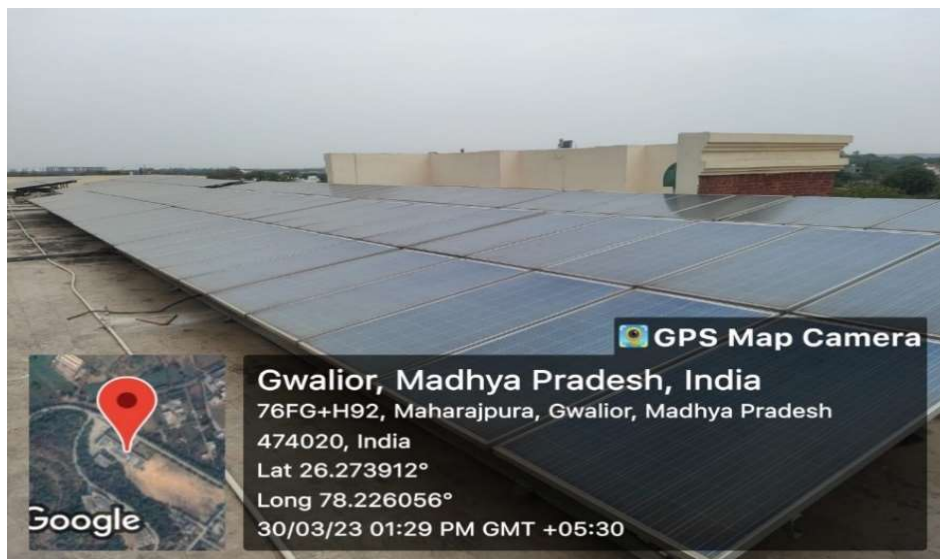
Solar Power Plant
